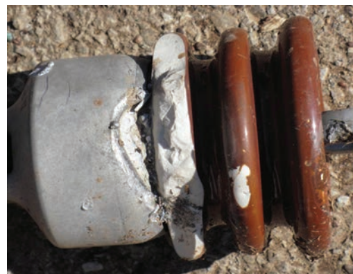
Fig. 4.65 Wire Insulation Damage
