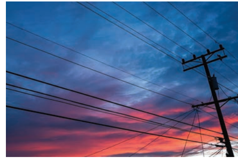
Fig. 4.50 Power Distribution Lines
