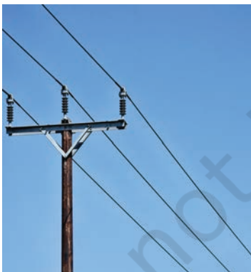
Fig. 4.54 Low Tension Distribution Lines (LT)
