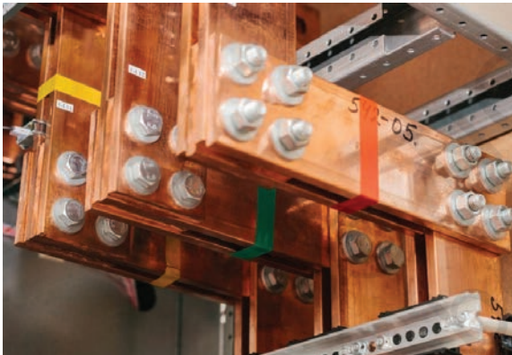
Fig. 2.12: A busbar for power distribution
