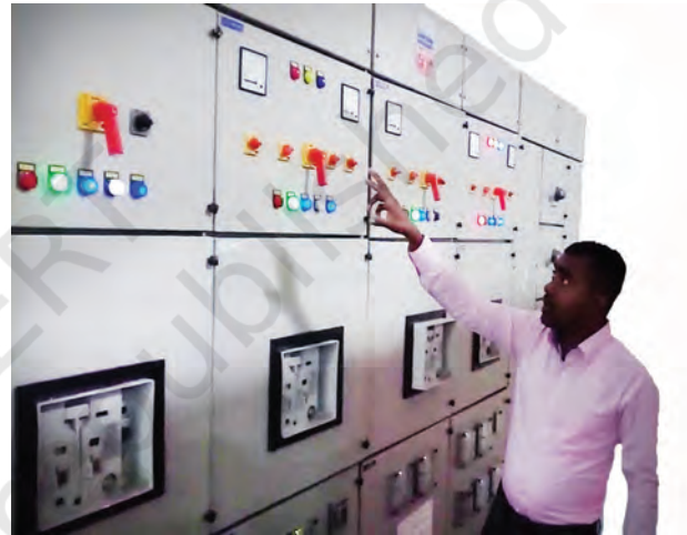
Fig. 1.44: Switchgear in the substation
