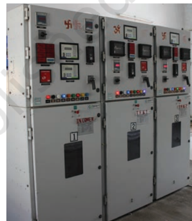
Fig. 5.5: Power panel board
