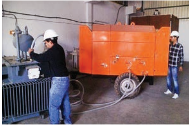
Fig. 11.19: Filling oil in a transformer using an oil filling machine
