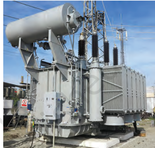
Fig.1.14: Transformer in the electrical substation
