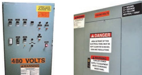
Fig. 11.9 (a) and (b): Written instructions and warning on a control panel
