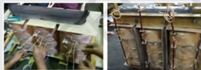
Fig. j: Making a series of connections of all the bundles of the primary coil. The terminals of the coils are connected in such a way that it forms a delta configuration.
