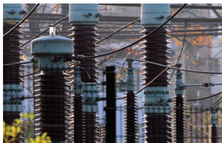
Fig. 10.2: Current transformer in an electrical sub-Station
