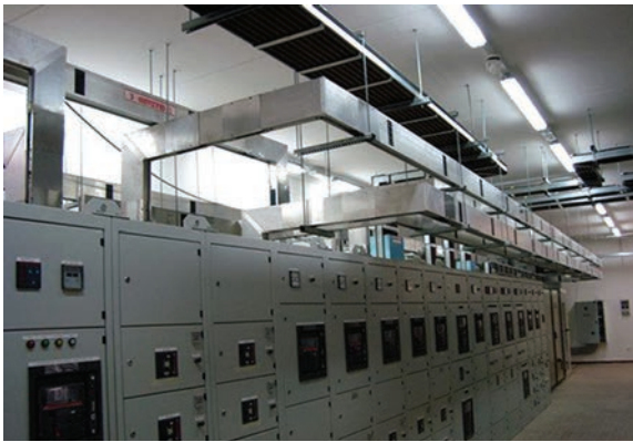
Fig. 2.11: Industrial application of a busway
