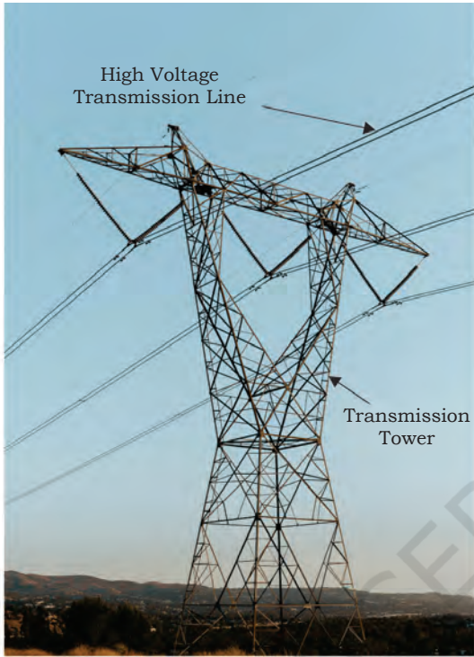
Fig.1.2: Transmission tower for transmission of electric power
