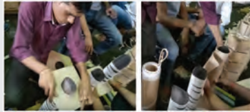
Fig. f: Insertion of insulation paper in the core of a three-phase transformer
