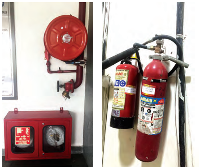
Fig. 5.1(a,b) Fire extinguishers
